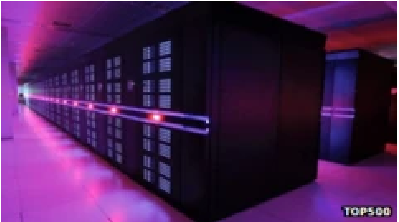
| Tianhe-2 uses a locally developed Linux-based operating system
