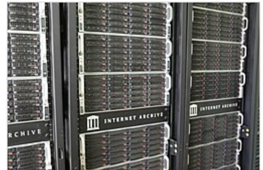
Servers at the Internet Archive headquarters in San Francisco
