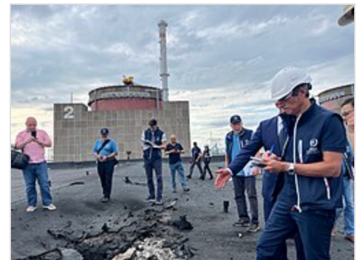
IAEA inspectors recording damage at Zaporizhzhia NPP
